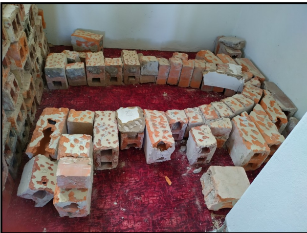
3. Bricks laid out in order as they were removed from the sacristy.
